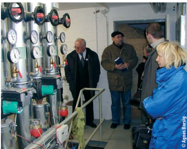
Exchange of experiences is one of RegioSustain's main objectives. Regular field trips with project partners to model initiatives - here a heating system based on the combustion of wood chips - probably are the most practical way to exchange and transfer best practices.
